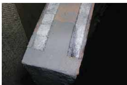
Figure 14 Asbestos panels inside fire door
