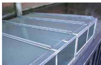
Figure 31 Chrysotile string on skylights
