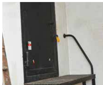
Figure 45 'Durasteel' composite steel and asbestos fire door
