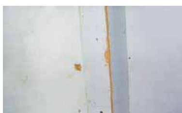
Figure 24 Chrysotile paper on fibreboard boxing
