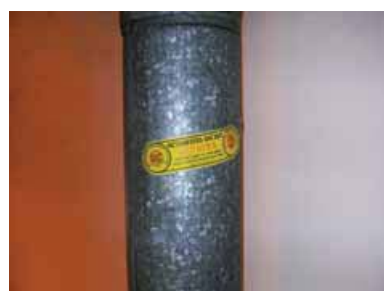
Figure 43 Metal clad gas flue containing chrysotile lining
