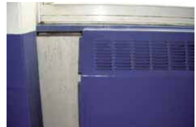
Figure 19 AIB behind school radiator unit
