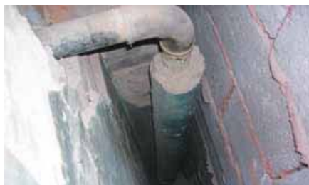
Figure 9 Lagged pipe in wall cavity
