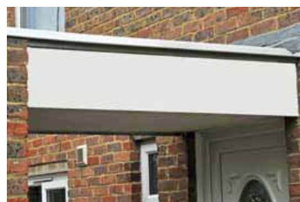
Figure 15 AIB panel in porch
