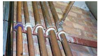
Figure 29 Chrysotile cloth on pipes
