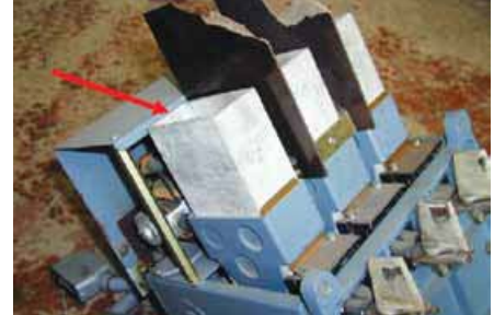
Figure 49 Electrical switchgear with asbestos flash protection
