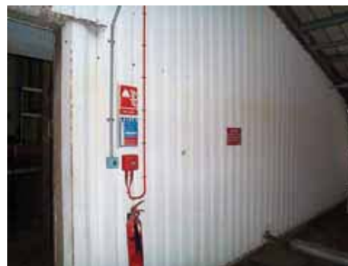
Figure 38 Chrysotile/bitumen coating under metal cladding
