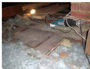
Figure 6 Loose asbestos used as loft insulation
