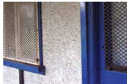
Figure 33 Chrysotile pebble-dash exterior wall coating
