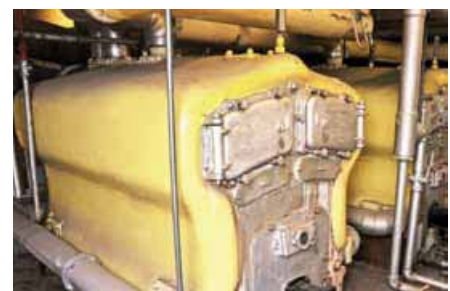
Figure 13 Amosite lagged boiler with hard plastic coating
