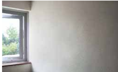
Figure 37 Asbestos textured coating on wall
