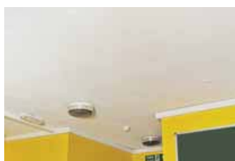
Figure 36 Asbestos textured coating on ceiling
