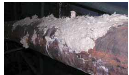
Figure 11 Amosite lagging in very poor condition on steam pipe
