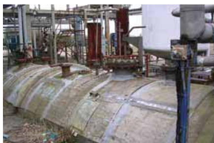
Figure 12 Lagging on large petrochemical vessel
