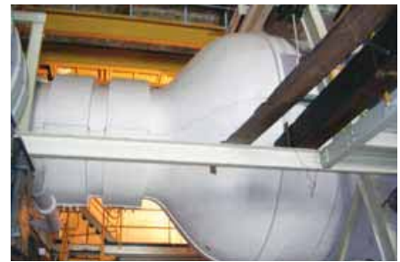
Figure 51 Vessel clad in amosite insulation
