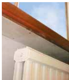
Figure 20 AIB panel between radiator and window
