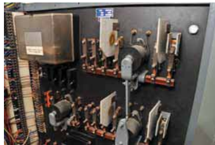
Figure 50 Open electrical switchboard with asbestos flash guards
