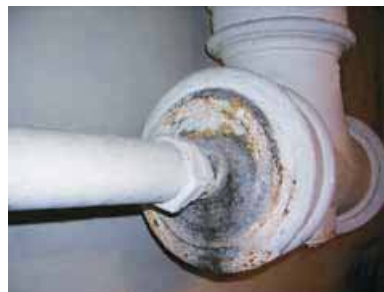
Figure 30 Amosite and chrysotile packing on waste pipes
