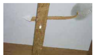
Figure 25 Chrysotile paper on strawboard ceiling panels
