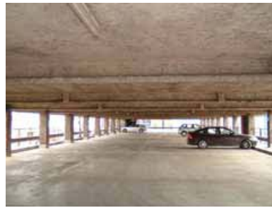
Figure 7 Sprayed limpet on car park roof
