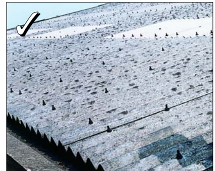
Asbestos cement sheets or guttering
