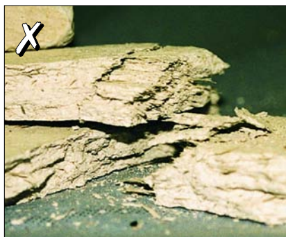
Damaged asbestos insulating board
